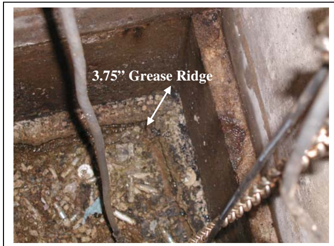
Sump Station 2 Wet Well
