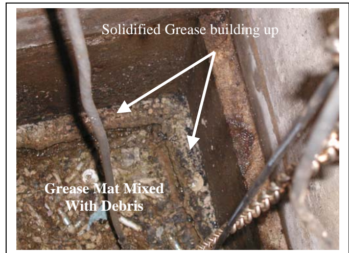
Inside Wet Well Sump 2
